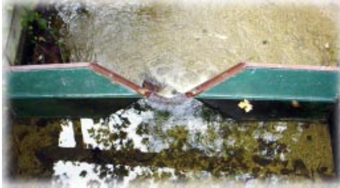
Weir at Main Stem flume.
